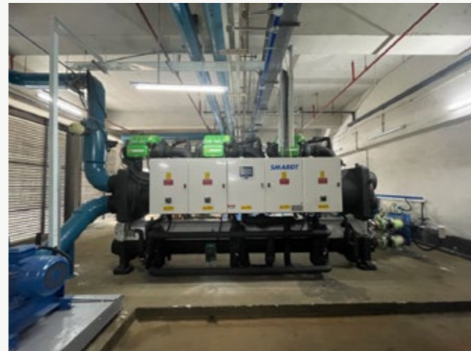
Novel integrated innovations and more sustainable refrigerants were also adopted to upgrade the centre's chillers to reduce energy demand.
